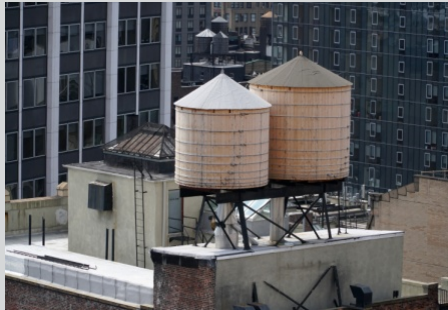
On-site water storage
